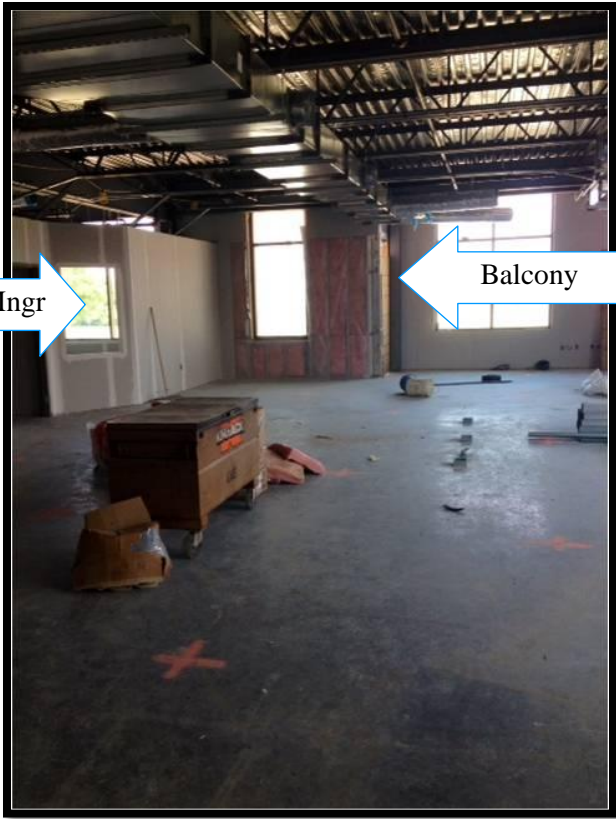
Looking Into Comm Center From Door near Lunch Room
